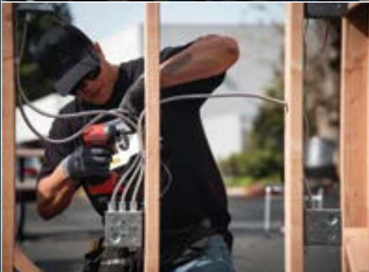
Residential Wiring: Adolfo Tinoco
